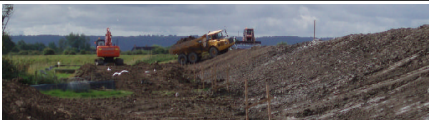
A recently completed new length of flood bank on the Congresbury Yeo in North Somerset, built further inland for long term security.
